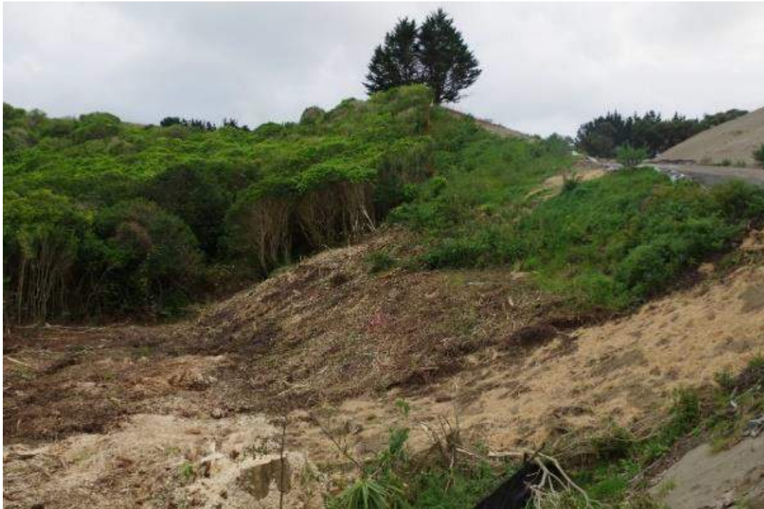
Figure 36: Upper and lower tracks exposed on western edge of expressway alignment (12 June 2015).
