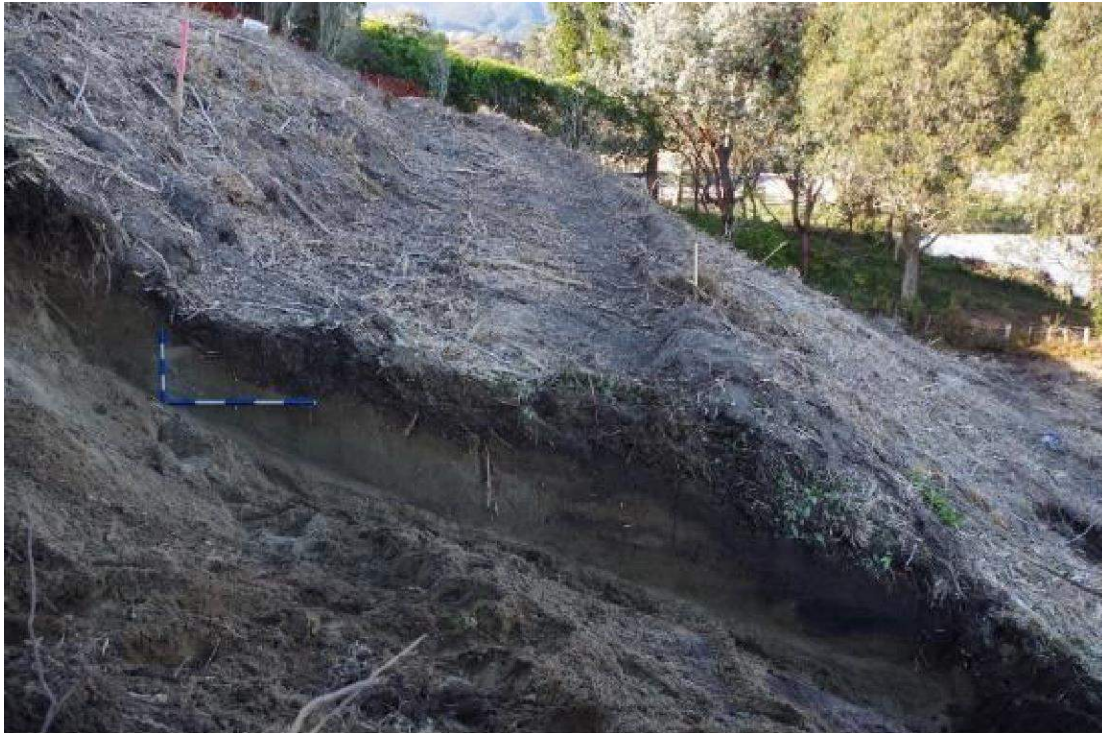
Figure 34: Upper track exposed in profile during haul road construction, scales 1.0+0.5 metres (25 August 2014).
