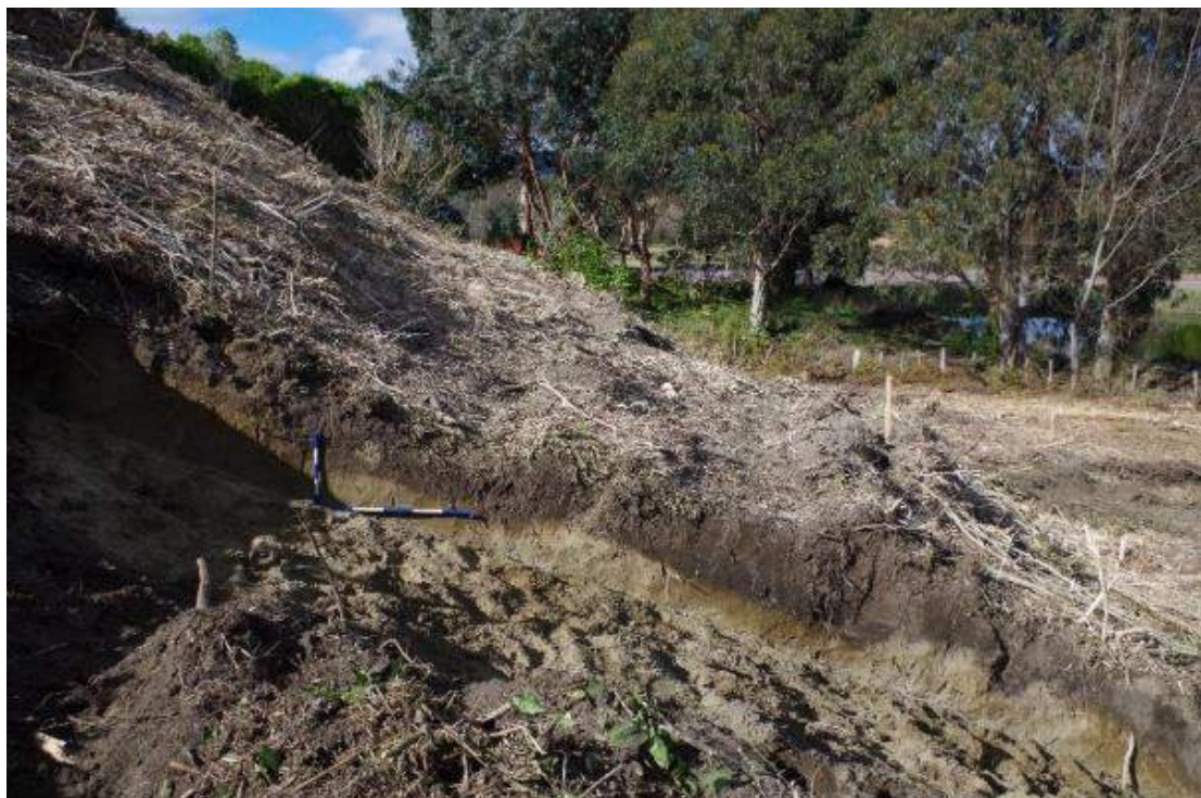
Figure 35: Lower track exposed in profile during haul road construction, scales 1.0+0.5 metres (25 August 2014).
